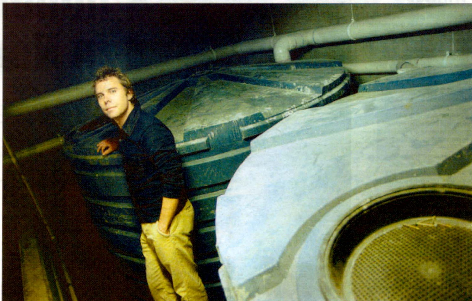
Luke Middleton with the water tanks he has incorporated into his building design.
