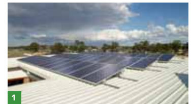
1. Sustainable houses give you the power to make a change
