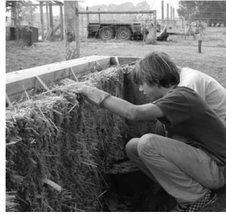
Woodleigh Grammar School Strawbale walls Architect: Luke Middleton from eme Design Pty Ltd Image: Scott Haskins
