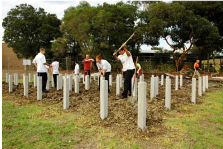
Figure 5 – students working on the foundations of the recording studio (Thornbury High School 2009)
