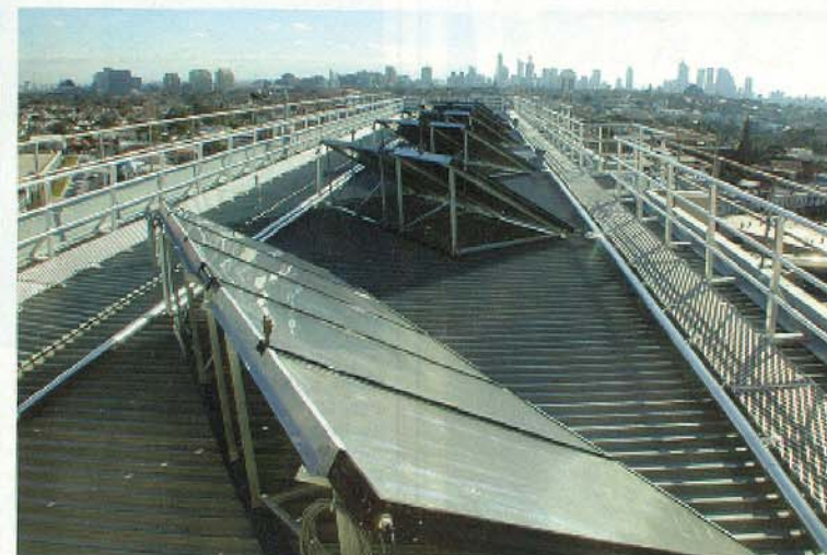
Solar panels for public-housing towers.
